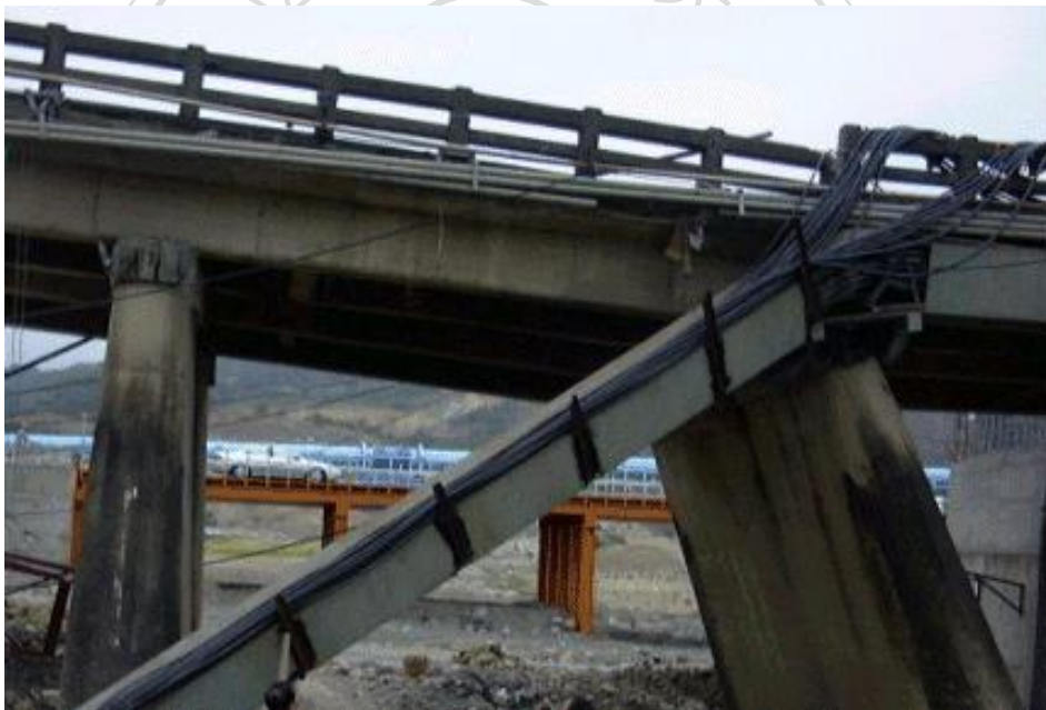
Figure 1.3. Broken bridge cut off communications cables
